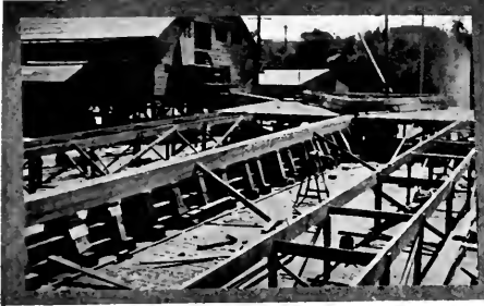
At Old Town, Tacoma, Babare Brothers, who have long been noted as producers of high class cannery tenders, purse seine boats and other fishing craft, are just completing a large extension to their plant.
